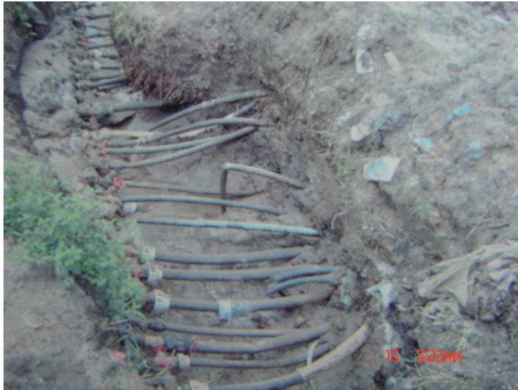
Figure 4: Illegal water connections in Dar es Salaam
