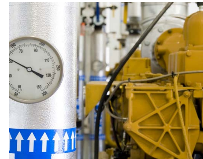
Inside a landfill gas recovery plant
