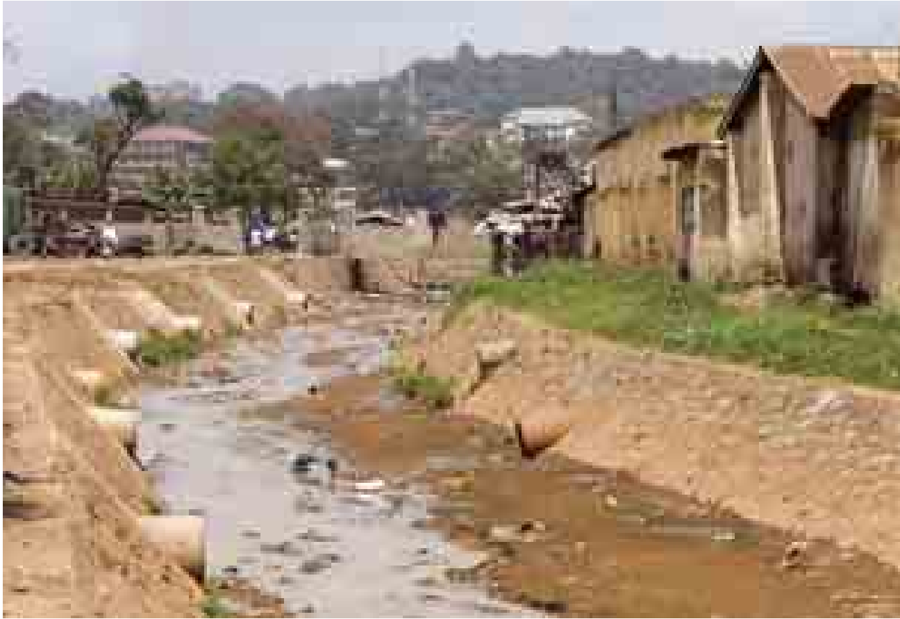
▲ Open sewer system in Kampala, Uganda. © Frank van den Bergh/iStockphoto
