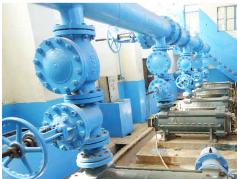
The booster station at Geed Deeble.
