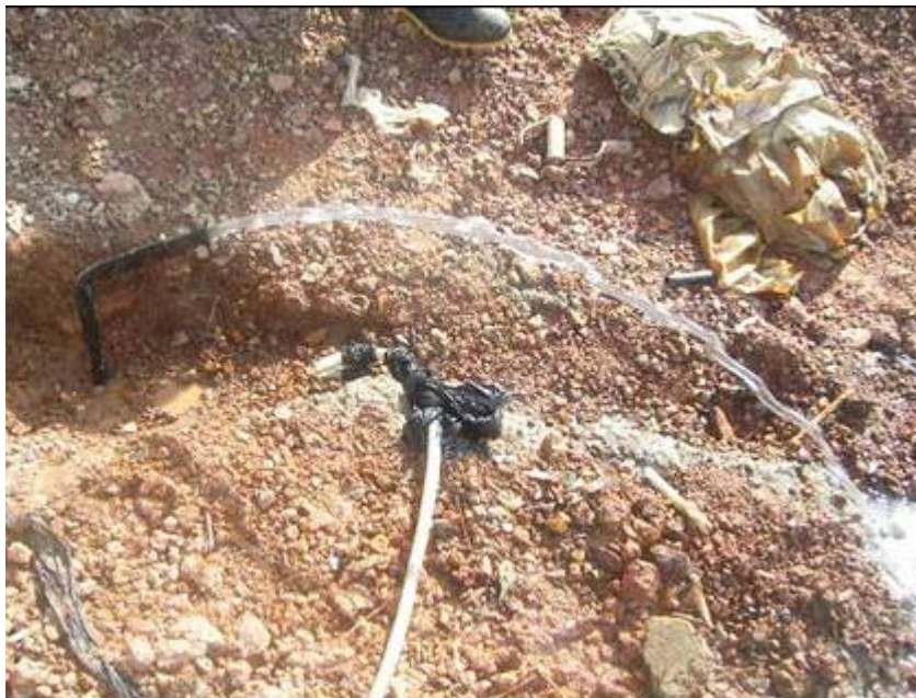
Plate 2: An illegal connection made onto the network
