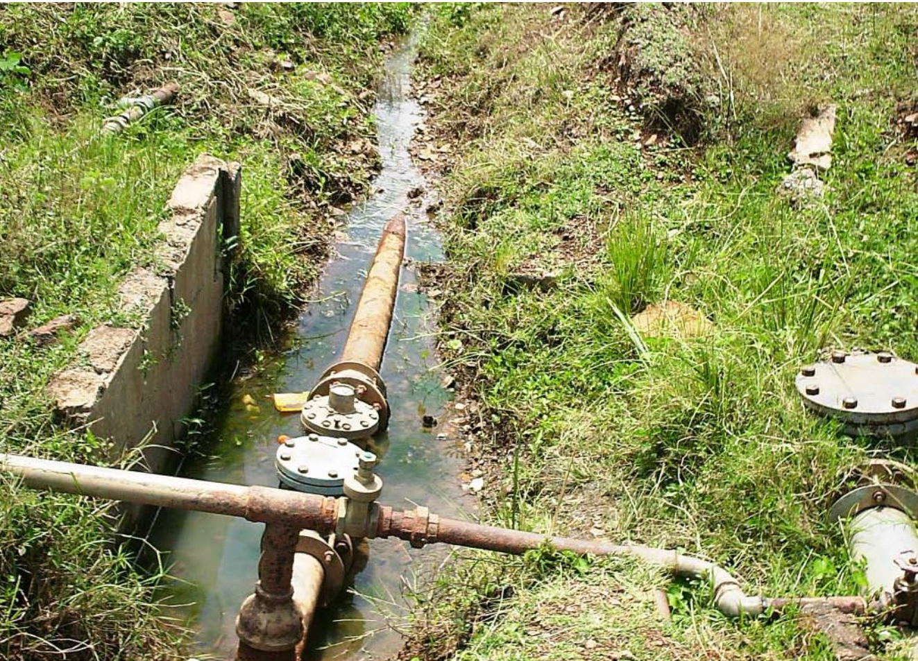
A leaking pipe. Photo © UN-Habitat
