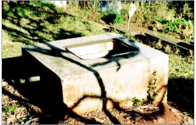
Plate 3. A vandalised inspection covers for a sewer drain. Stones and other objects may fall in and block the drain.
