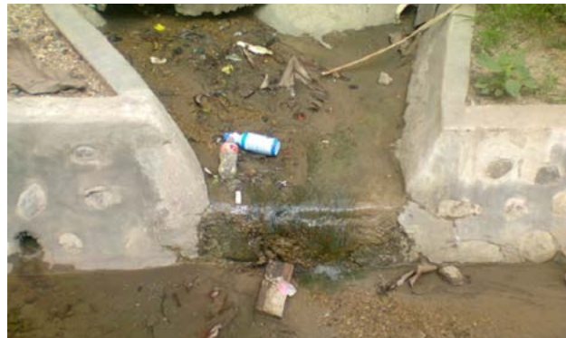
Drains blocked with soil and other waste materials in the Gordens Area Photo © Goije, B., Kioma, T., Bobora, N., Bomai, A. and Kamaso, D. (2012)
