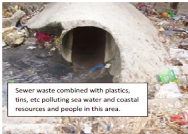
(Left) Children washing in open drains in the Boroko creek (Right) Illegal Water Connection in National Capital District's 8 Mile Settlement Photo © Poua, R. and Malu, J. (2012)
