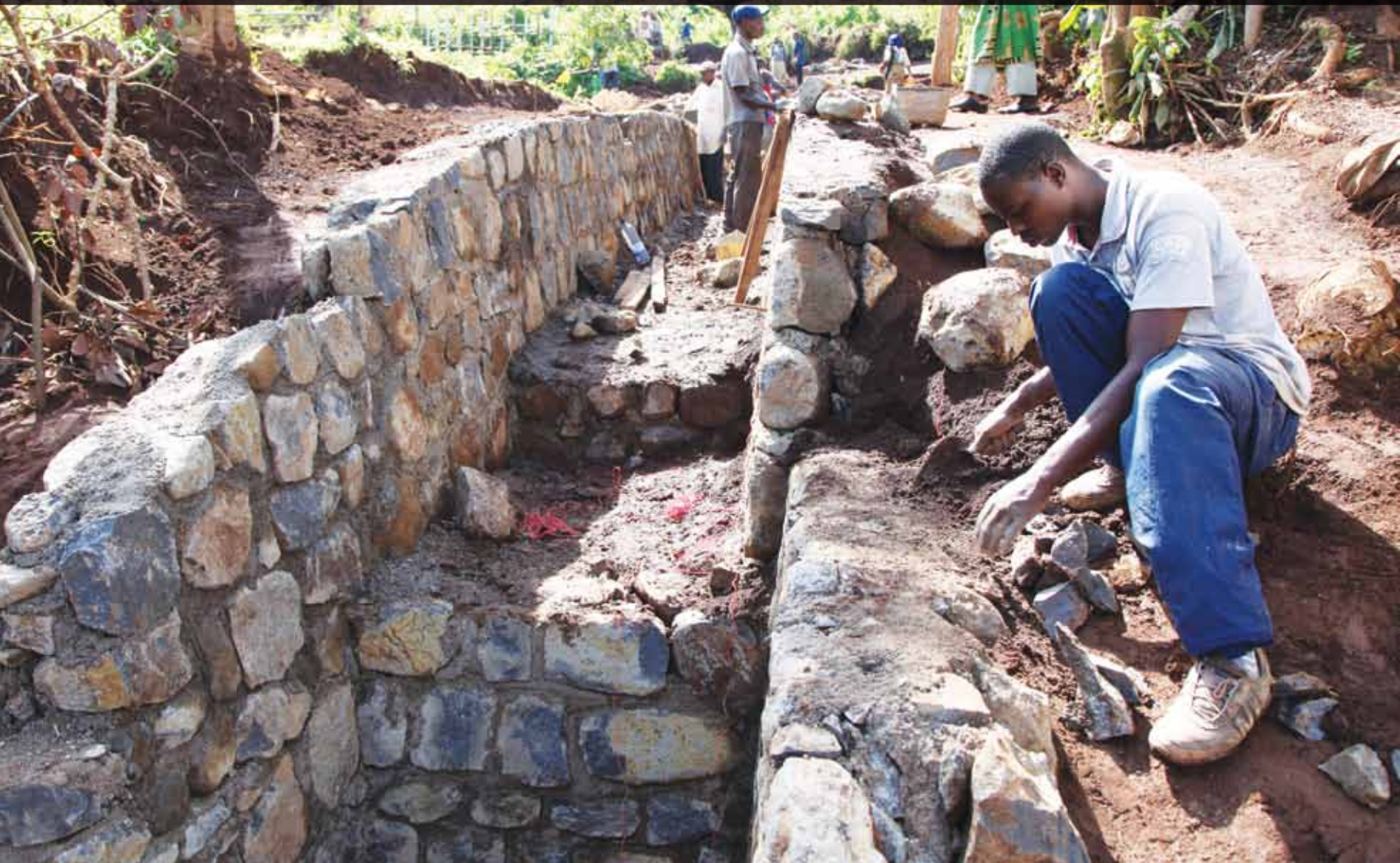
Construction of a water tunnel supported by UN-Habitat and ONE UN in Rusizi, Rwanda 2012 © UN-Habitat, Julius Mwelu
