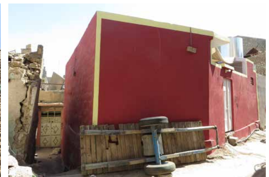
FIGURE 128. Ongoing reconstruction in the Old City Currently, local residents engage in the reconstruction of private houses (UNESCO, Giovanni Fontana Antonelli, May 2018).
