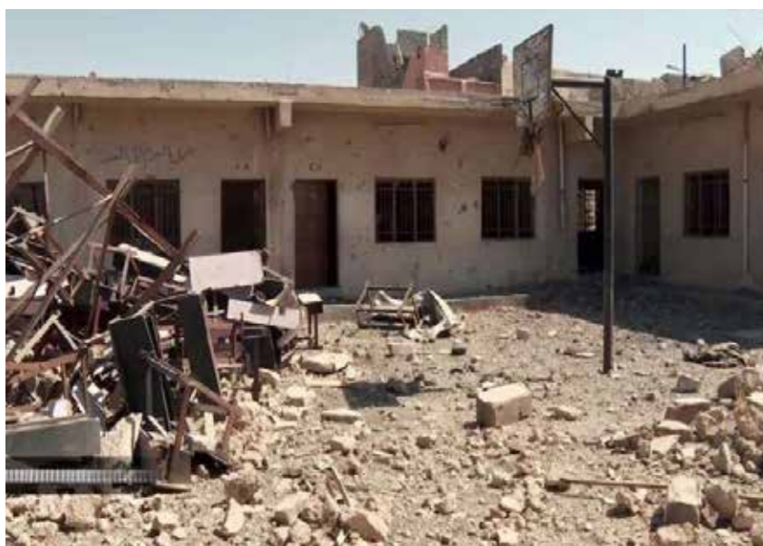
FIGURE 136. Damage to one of the 37 schools in the Old City Schools in the Old City suffered from the extensive fighting.
