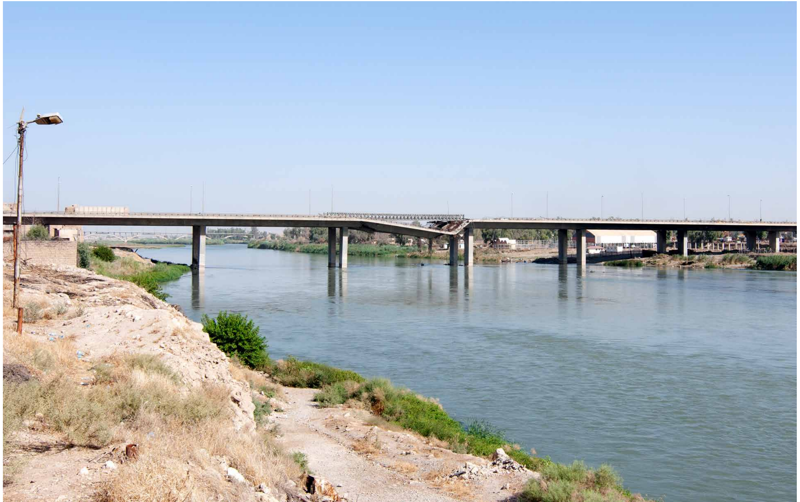
FIGURE 38. The Fifth bridge over the Tigris River has been partially destroyed. A temporary Irish crossing has been put in place to facilitate some freedom of movement (UN-Habitat, Jan Willem Petersen, November 2018)
