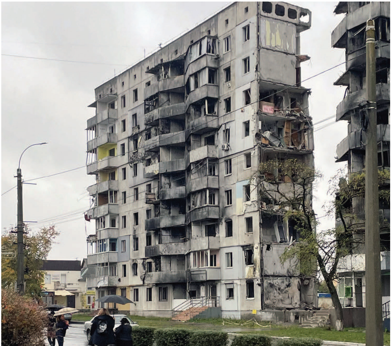
A war-damaged residential building in Borodianka, Kyiv Oblast © UN-Habitat Ukraine
