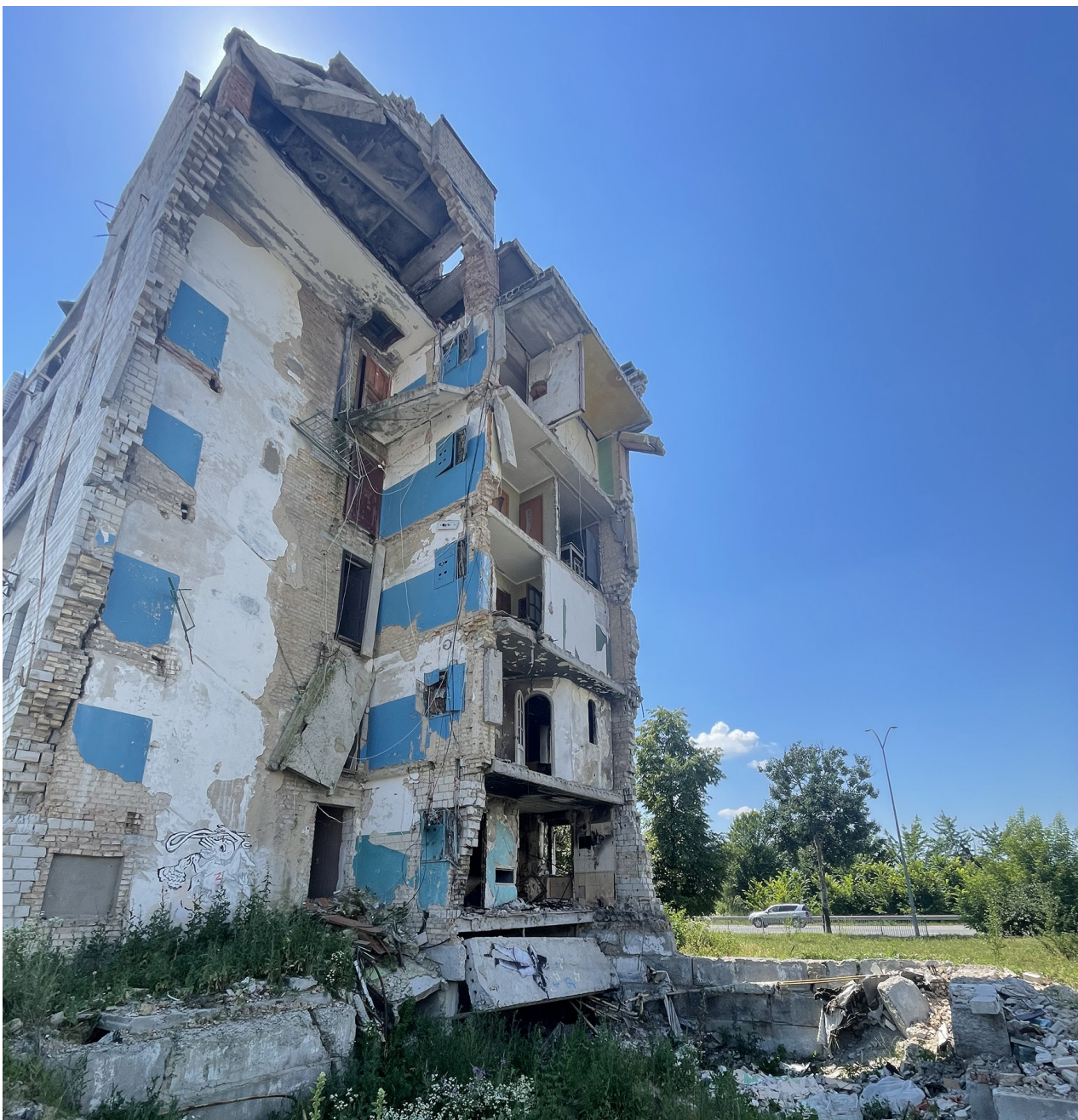
Heavily destroyed residential building © UN-Habitat Ukraine
