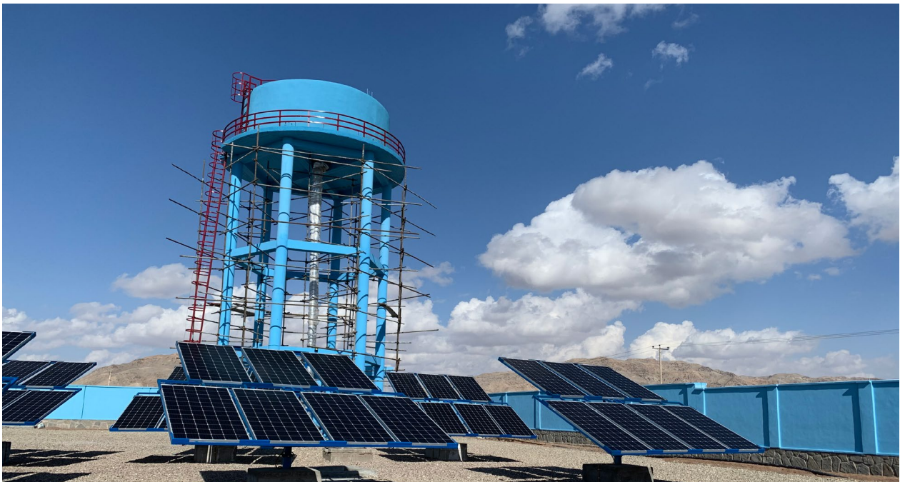
Solar-powered water supply facility in Saadat Township in Herat province. June 2020. ©UN-Habitat
