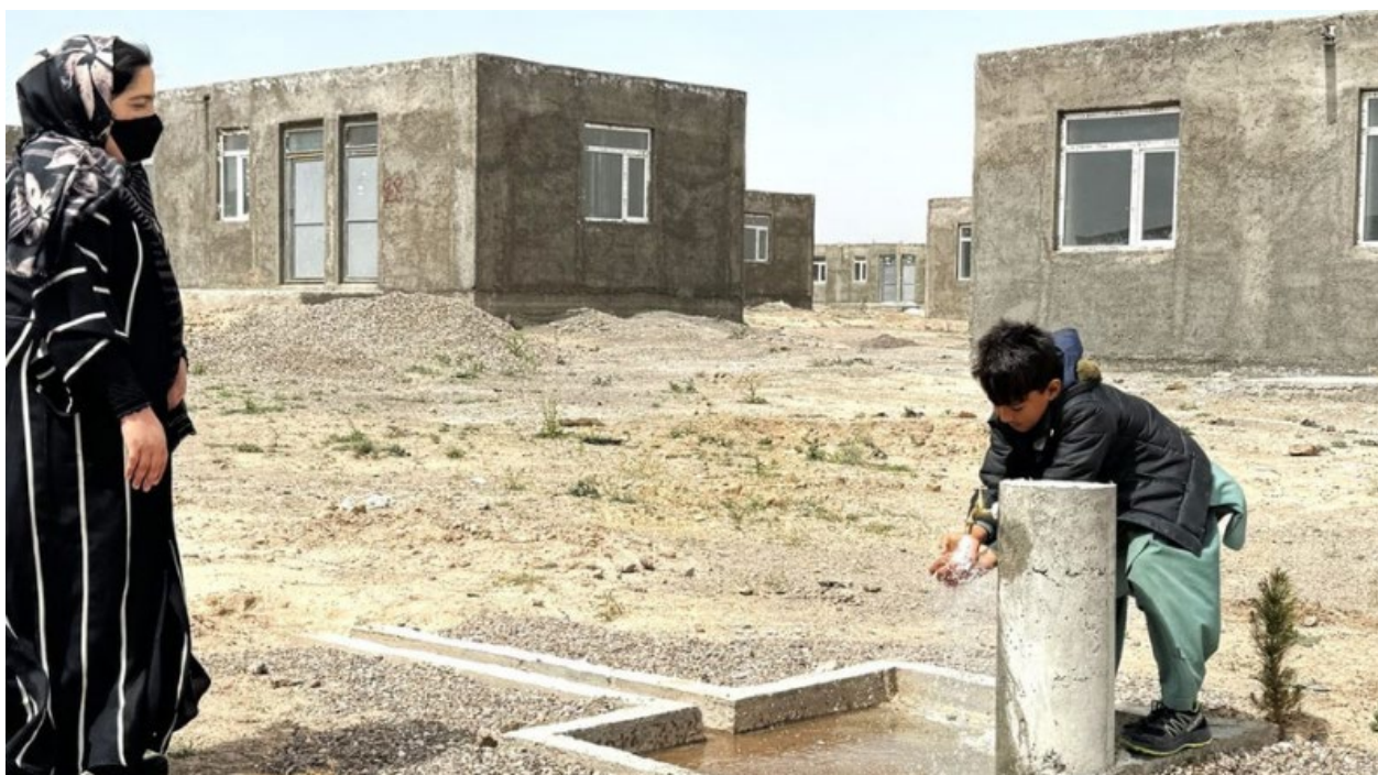
Some houses and water services were available during construction in Herat. March 2020 ©UN-Habitat
