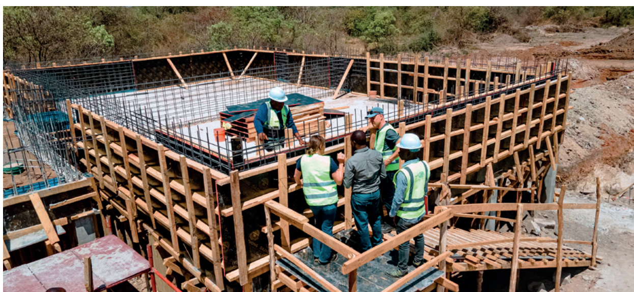
Kahama Water Supply and Sanitation Authority and Hamburg Wasser peer colleagues discuss design details for a rainwater treatment plant under construction in the United Republic of Tanzania. Credit: Magige Marwa/Kahama Water Supply and Sanitation Authority
