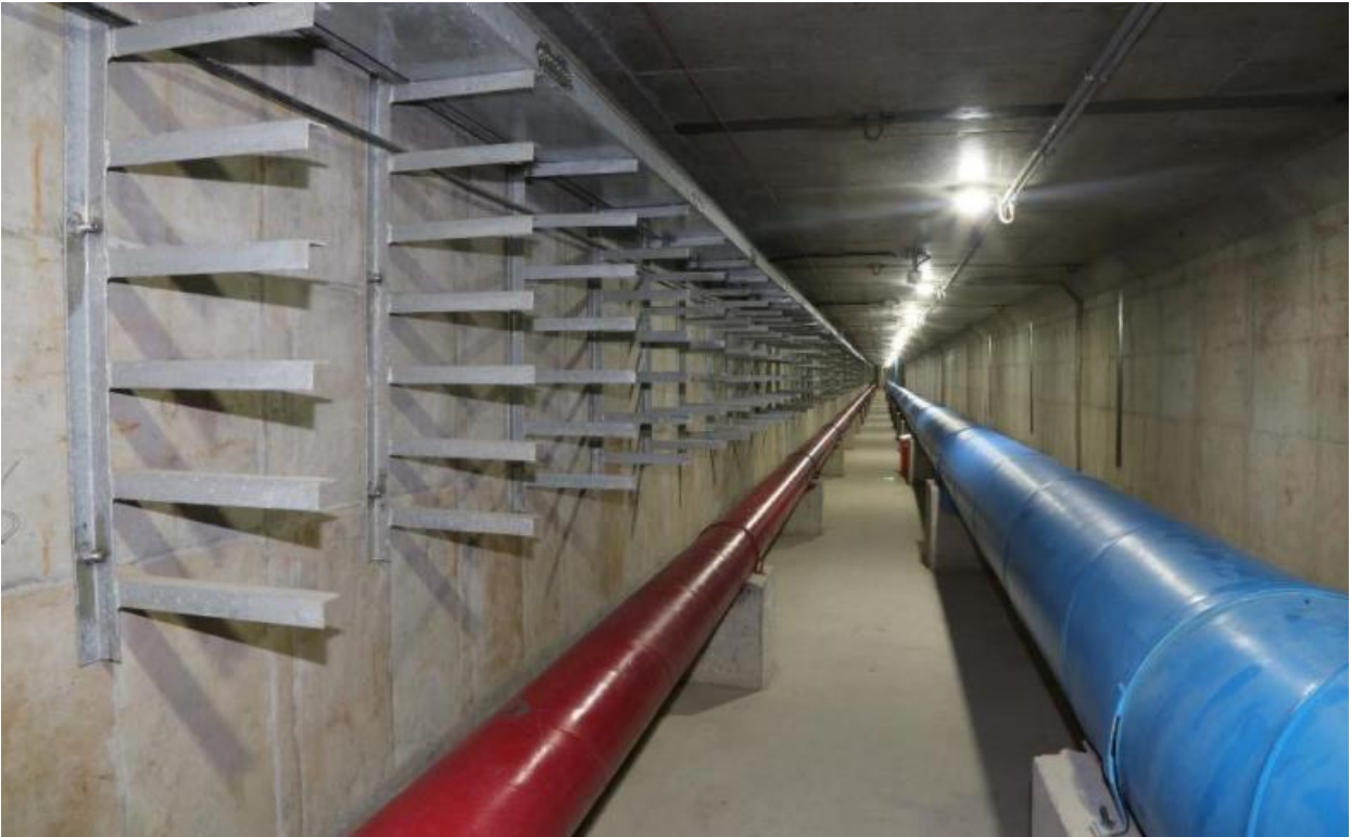
Figure12 Beijing Future Science City's Core Area of Comprehensive Pipeline Corridor
