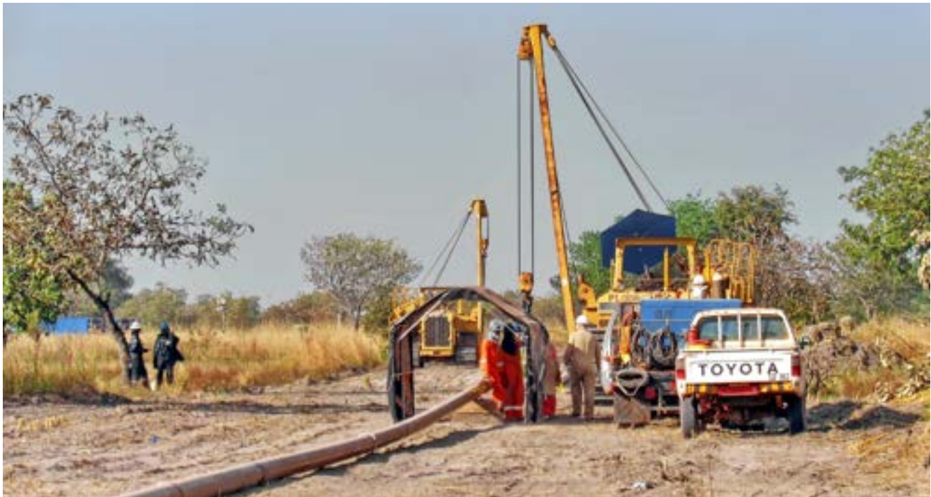
Installation of a new oil pipeline in a rural area in sub-Saharan Africa in Doba, Chad. © Shutterstock
