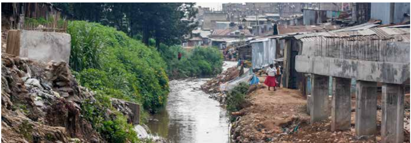
The construction of the bridge in Mathare slum, Nairobi, Kenya in 2016 © Julius Mwelu_UN-Habitat
