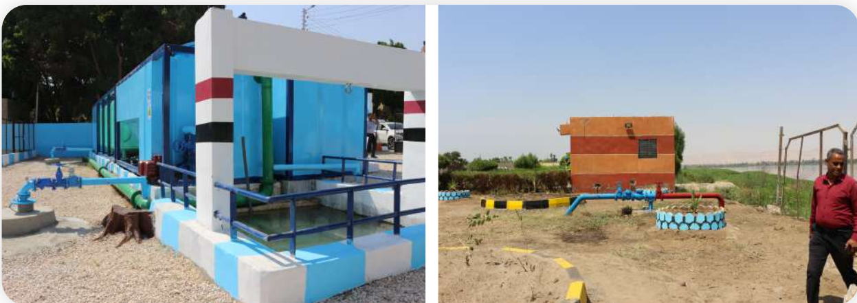
Figure 34 Pumping Wells of RBF Units in Egypt
