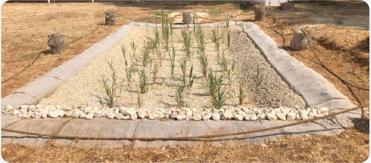
Figure 38 Constructed Wetland, Bekaa, Lebanon
