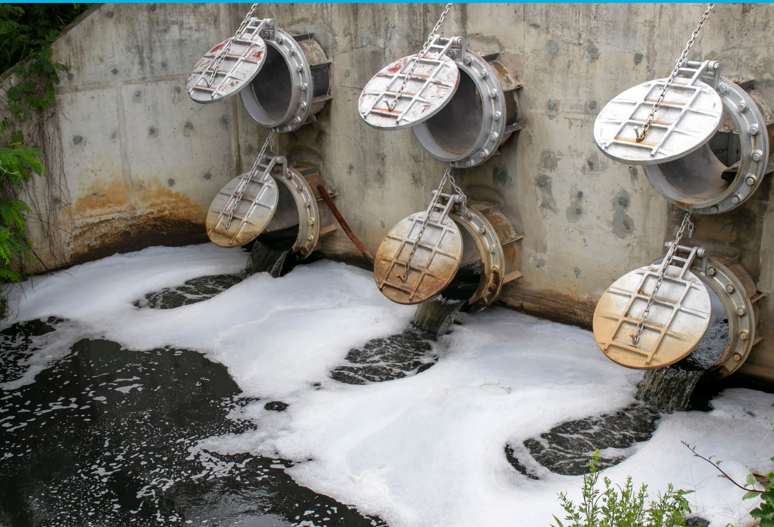
Concrete outfall structure with multiple flap gates. Photo: Siyanight/Shutterstock
