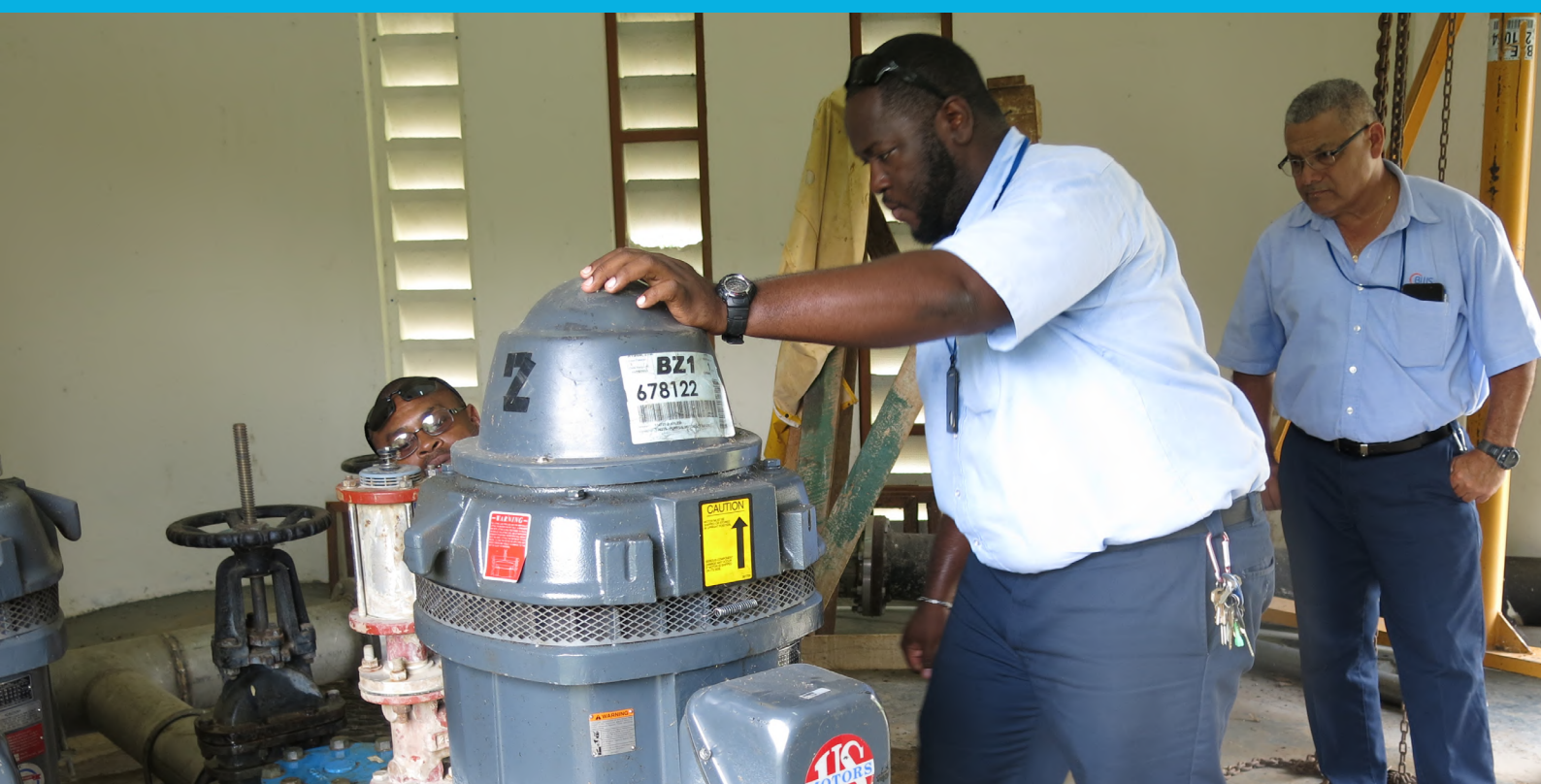
Inspecting of a vertical turbine well pump by a Belize Water Services team. Photo: Belize Water Services
