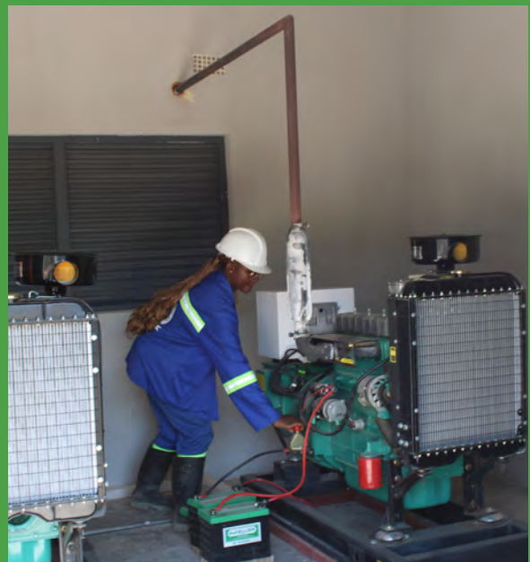
Jane Mulenga, a Wastewater Treatment Plant Operator, oversees the machinery that converts waste into electricity.
