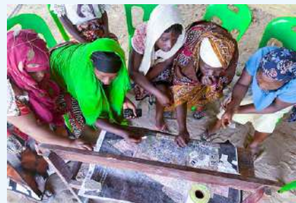
Women were trained in several trades from carpentry to bricklaying, enabling them to build their own houses © UN-Habitat Mozambique
