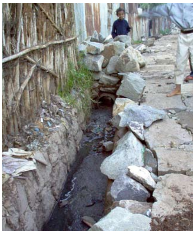
A typical drainage channel in the inner-city slums. Photo: © AAGG
