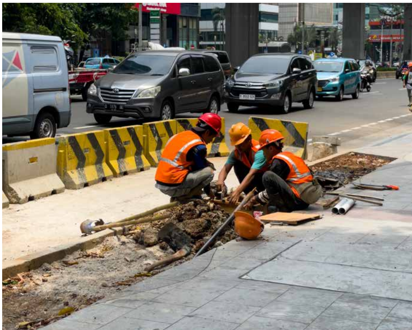
Sidewalk repair in Jakarta, Indonesia © Shutterstock
