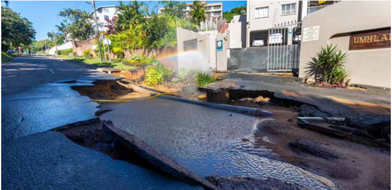
Damage to infrastructure caused by natural disaster, Durban, South Africa © Shutterstock
