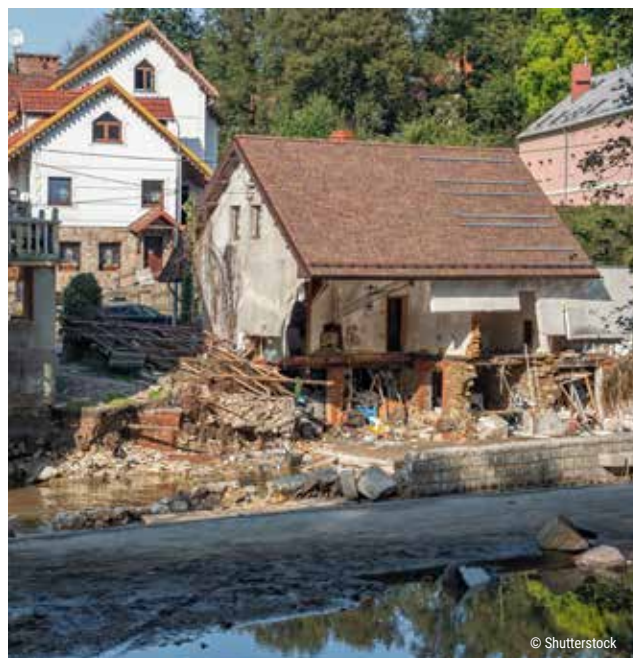
Ladek Zdroj, Poland - September, 17, 2024: Biala Ladecka riverbed, flooded and destroyed houses, destroyed river bank, two days after the flood wave passed through the city. View from Kosciuszki Street/Shutterstock
