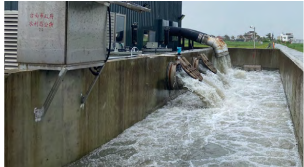
△ View of the Pumping System of the flood storage pond in operation
