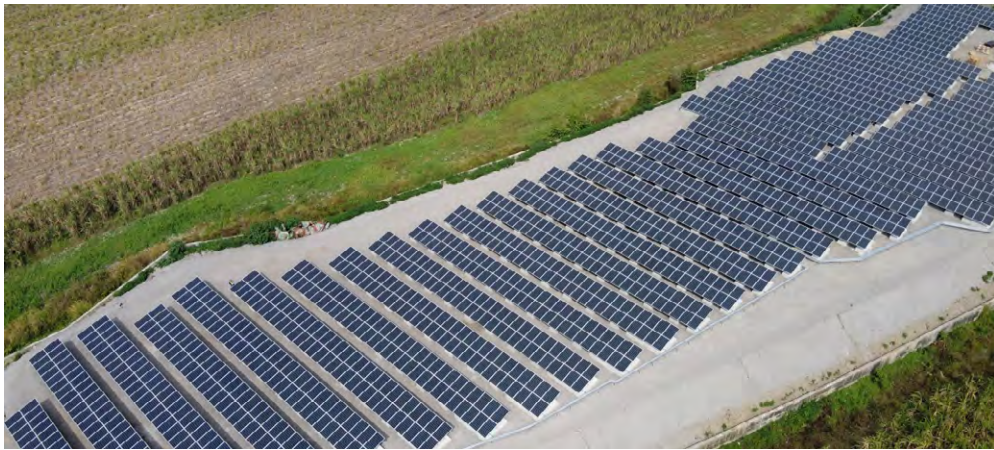
△Houbi District Jingliao Landfill Power Plant
