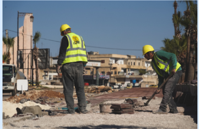
UN-Habitat and UNDP improved Dara'a streets, repairing sidewalks, asphaltting 985 meters, and adding solar lights. This benefited 18,000 residents and 50 shops. © UN-Habitat.
