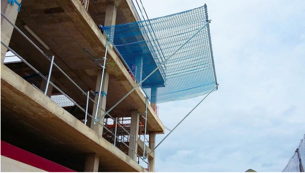
Safety nets, accessible from: safesmartaccess.com.au/safety-net-fans , accessed on 10/01/23
