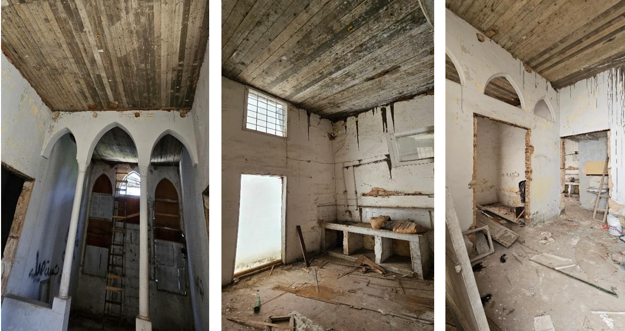
Figure 6: Images of Re_212 showing the building and its internal damages (UN-Habitat, 2023)
