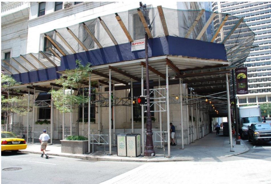
Overhead protection, accessible from: https://superiorscaffold.com/customizing-your-overhead-protection-the-ritz-carlton-philadelphia-pa/ , accessed on 10/01/23
