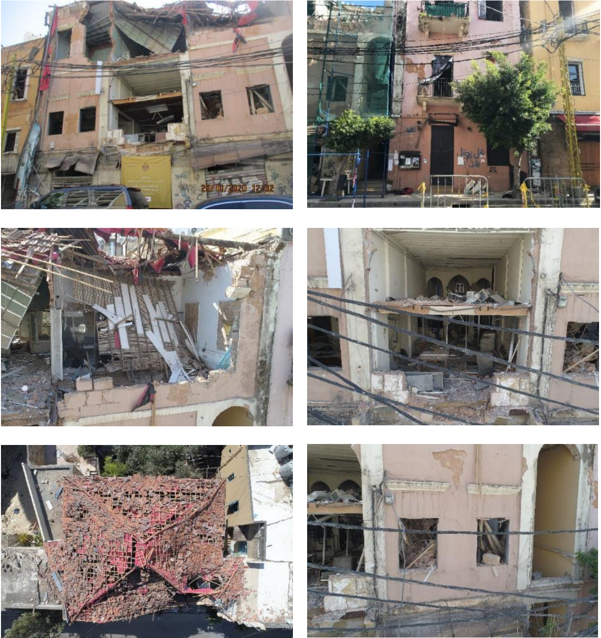
Figure 8: General Drone Images of Re 643-644 showing the building and its damages from different angles (DGA,2020)
