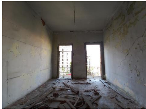
Figure 7: General Images of Re_425 showing the building and its internal damages (LDRS, 2023)
