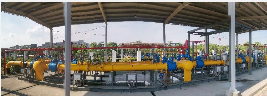
Figure 8 Natural Gas Station of Pu'nan Area in Songjiang
