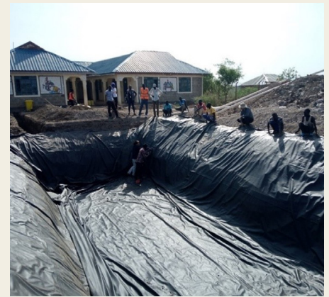
Daiken and construction team laying the geo-membrane for the underground water tank. © UN-Habitat
