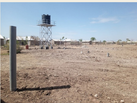
Completed underground water tank, with an erected elevated water tank in the background. © UN-Habitat
