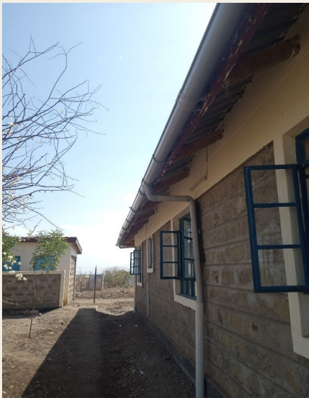
Rainwater collection gutters and downpipes. © UN-Habitat
