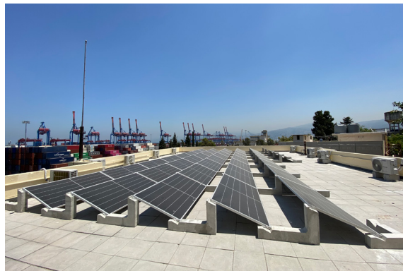
UN-Habitat installs 20 kWp photovoltaic and solar heating systems as part of its post Beirut blast rehabilitation efforts of the National HIV/TB Centre ©UN-Habitat
