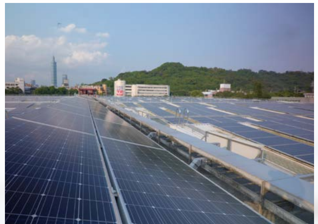
► Solar photovoltaic system installed in water.
