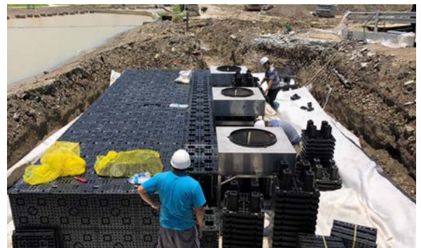
► Rainwater tank at Hsinhsin Park.
