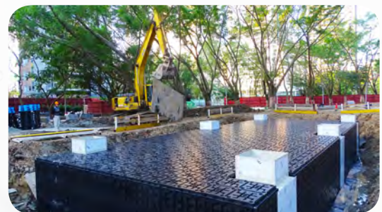
▲ Rainwater harvesting at Xiangshan Park
