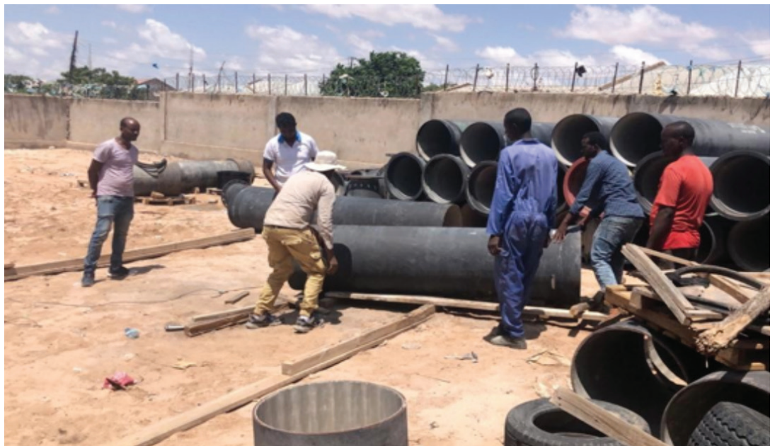
Figure 25: UN-Habitat completed the 23 kilometre long main transmission line between the Ged Deeble wellfield and the Hargeisa water reservoir.
