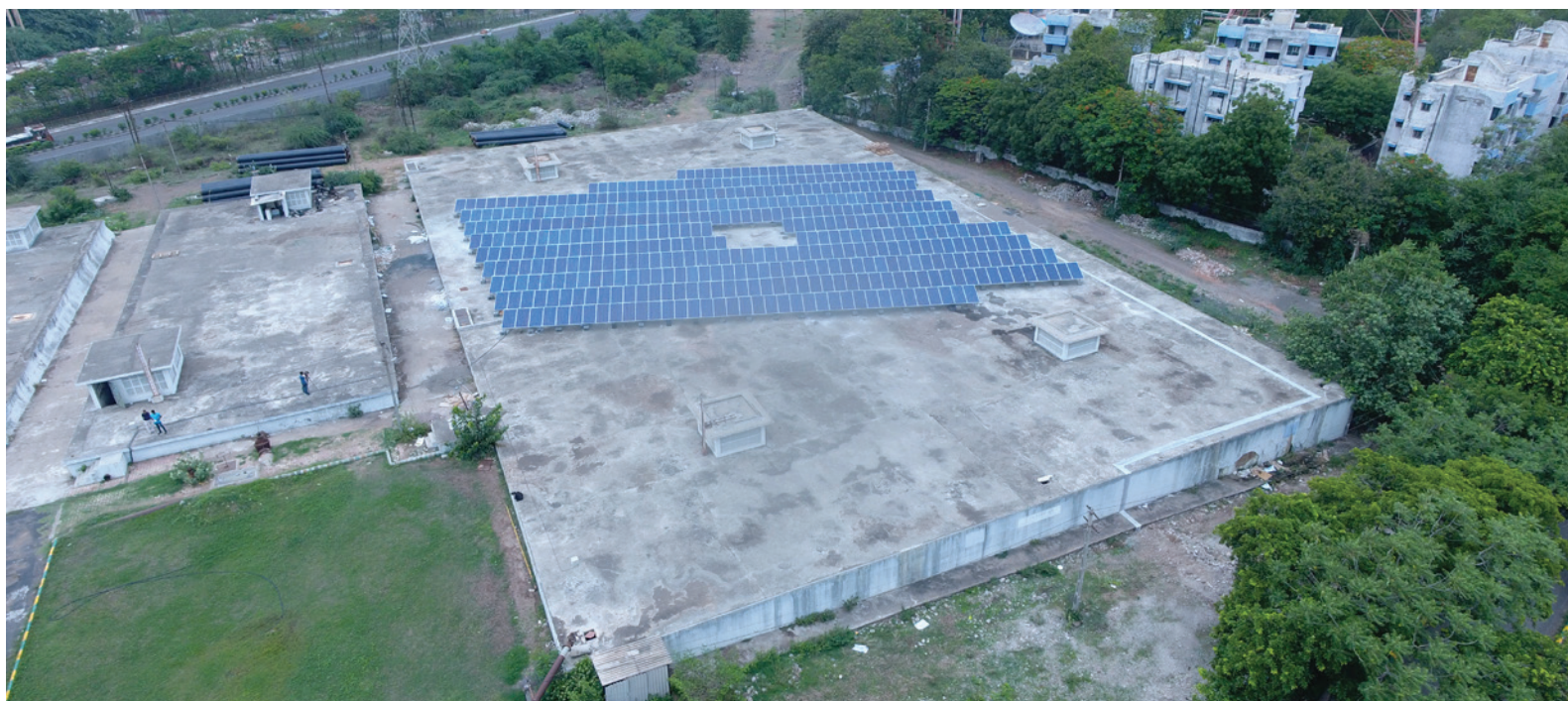
Rajkot, India, and Urban-LEDS project city, has installed a 145kWp solar PV system to help power its Aji water treatment plant
