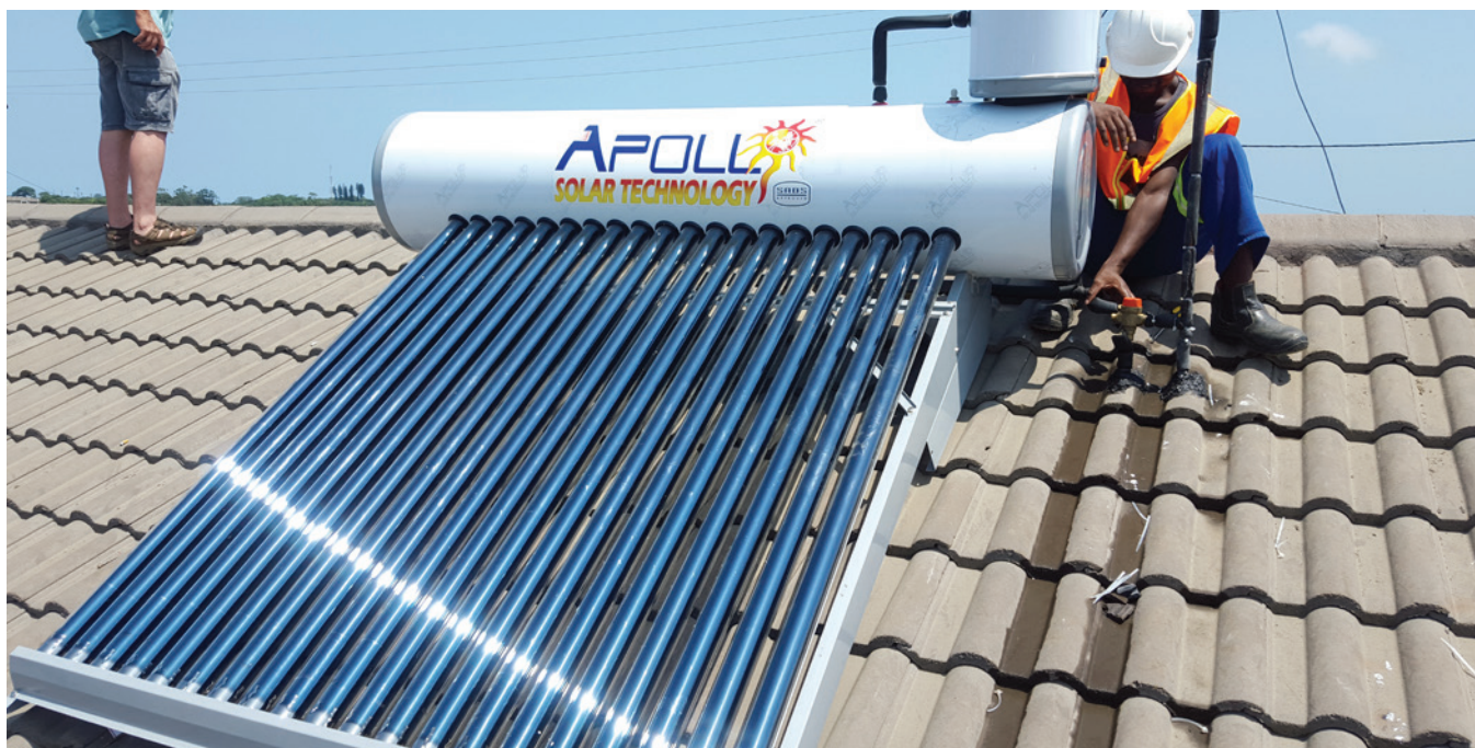
Solar water heaters save electricity and money – here installed on Groutville Care Homes in KwaDukuza, South Africa, as a pilot project implemented by Urban-LEDS
