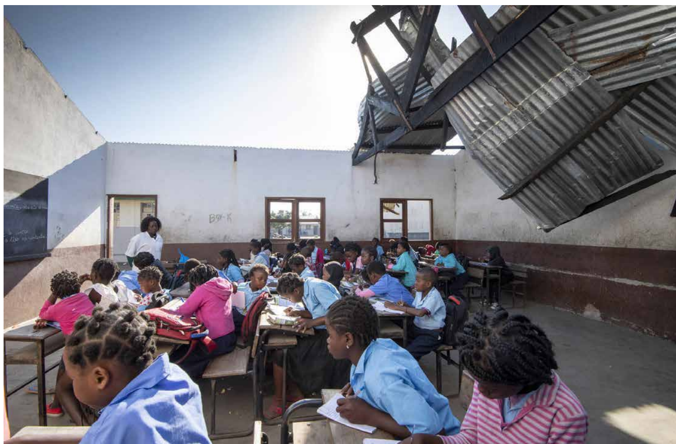
A school affected by Cyclone Idai in Mozambique. © UN/Eskinder Debebe
