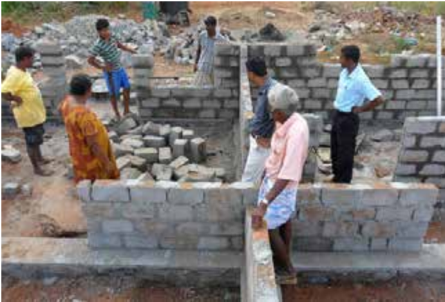
UN-Habitat engineers providing technical advice at Mrs.K.Karunakaran's house construction site, Vavuniya North. © Krishnarany Sinnapalani/UN-Habitat
