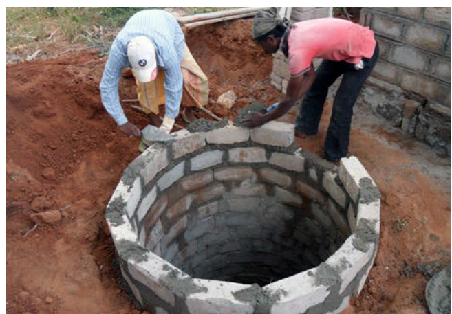
Toilet soakage pit under construction in Palaikkuli, Musali DS division in Mannar district with the home owner, Mr M H A Cader assisting the mason. © A.J.A. Thivakar/UN-Habitat
