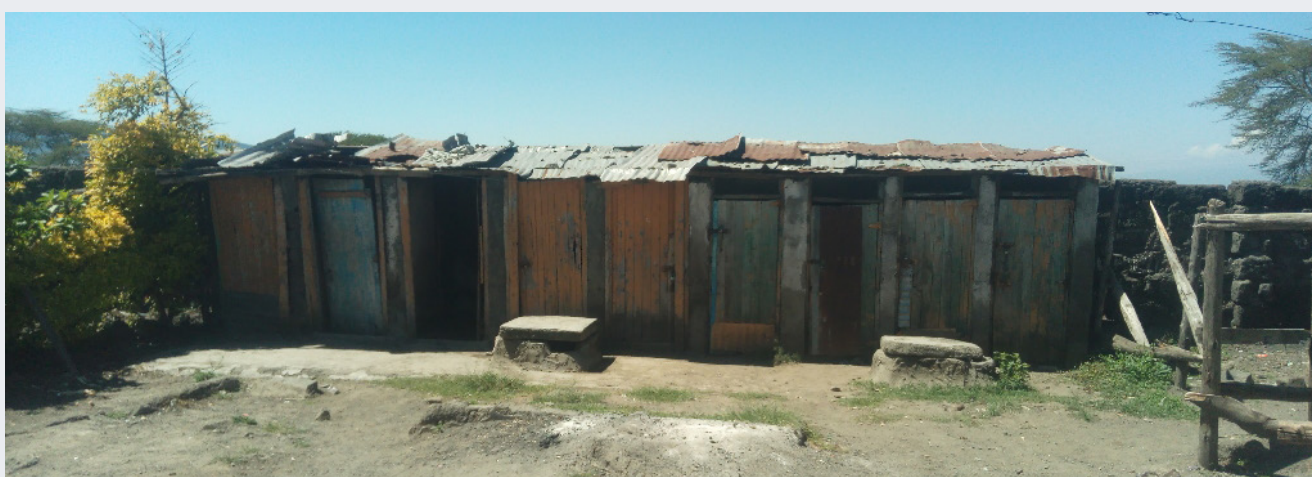
Figure 24: Poor conditions of Sanitation facilities in Bondeni
