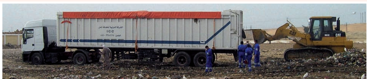
Photo 8.4 Tracked loader helping an empty articulated truck to move off the waste
