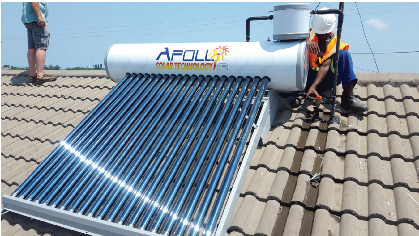
Solar water heaters save electricity and money – here installed on Groutville Care Homes in KwaDukuza, South Africa, as a pilot project implemented by Urban-LEDS
