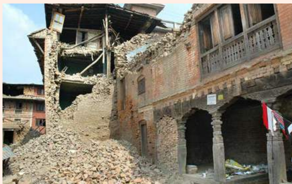
Houses, workshops, and community buildings damaged by the 2015 earthquake in the historic town of Bungamati, Nepal. 2015. Source: Shelter Cluster Nepal.
