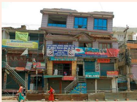
Individual building failure. Top story pancaked onto the three lower stories. Source: Shelter Cluster.
