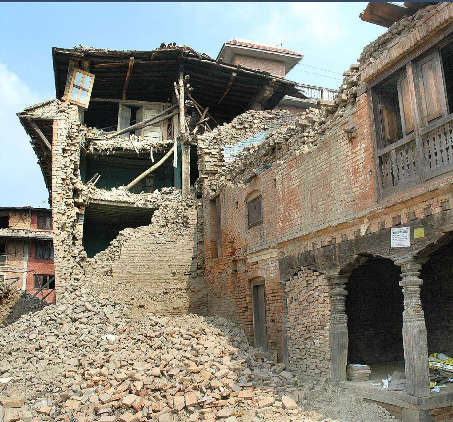
Houses, workshops, and community buildings damaged by the 2015 earthquake in the historic town of Bungamati, Nepal. 2015.
