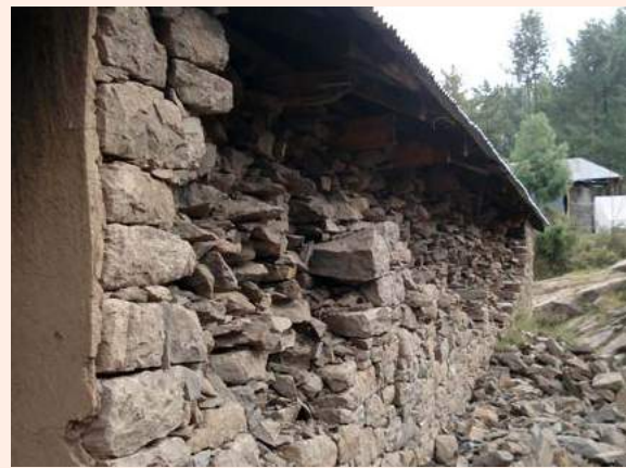
Earthquake damaged wall showing typical pattern of delamination. Pakistan. Source: GOAL Ireland.
