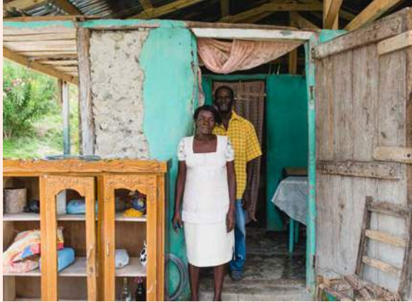
Typical rural house damaged by Hurricane Matthew. Haiti. Source: CRS.
