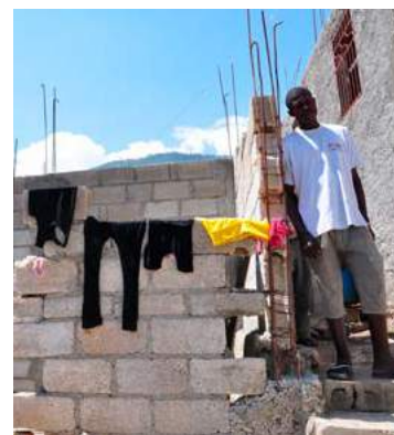
The majority of households in Haiti have very low incomes and reconstructed their homes without financial or technical assistance, reinstating or increasing their disaster risk. Source: UN-Habitat.
