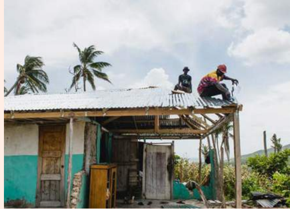
A mobile technical assistance team carries out repairs and strengthening on a damaged verandah roof. Source: CRS.
