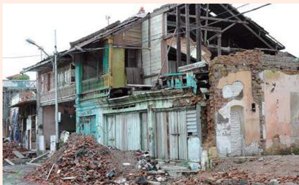
Historic shop houses damaged by 2009 earthquake in the centre of Padang, Indonesia. Mainly absentee property owners. Source: UN-Habitat.
