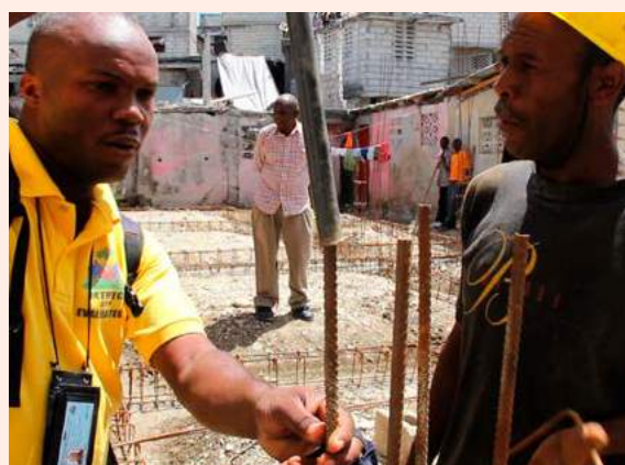
Government engineer on site in Delmas 32 explaining steel size information to local masons. Haiti. Source: J/P HRO.
