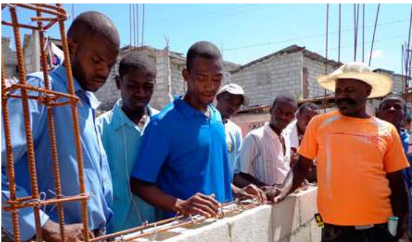
Visit to demonstration house and information event to learn safer construction standards and practical application. Source: Internews.
