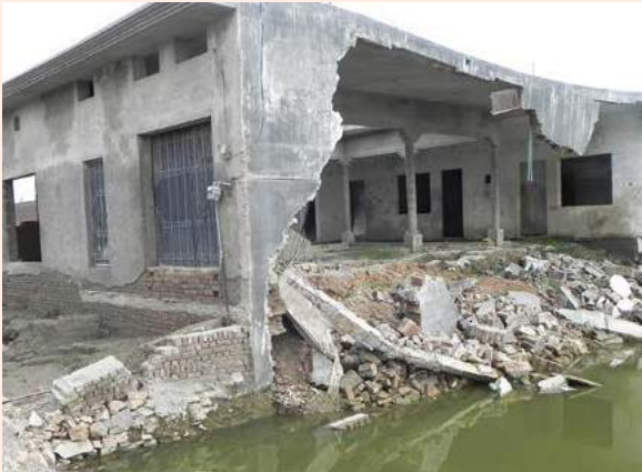
Standing water damage to concrete and brick masonry building. Source: UN-Habitat.
