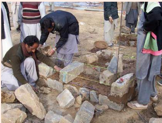
Training masons in traditional earthquake resistant stone masonry techniques. Pakistan. Source: GOAL Ireland.
