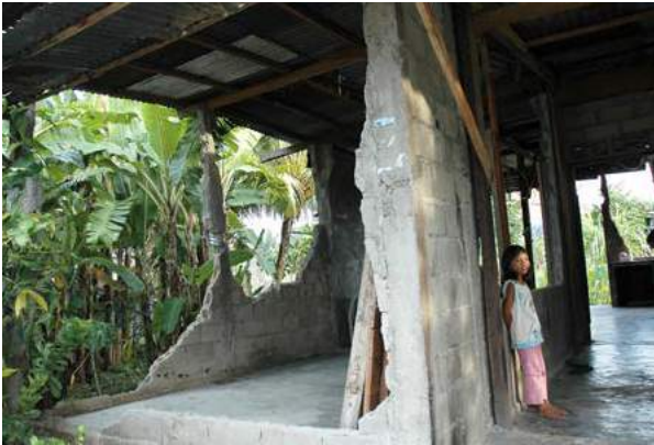
Children playing in unsafe damaged buildings, out of school after disaster and uncertain of their homes and futures. Indonesia. Source: UN-Habitat.
