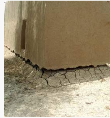
Low strength mud masonry. Difficult to develop standards to achieve resistance to flood or earthquake hazards. Heavy mud masonry buildings perform well on thermal and cost criteria. Source: UN-Habitat.
