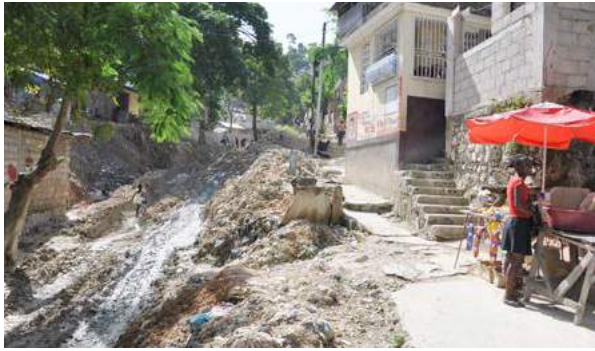
Ravine in informal neighbourhood of Campeche, Port au Prince, Haiti after the 2010 earthquake, before improvement measures. Source: UCL.
