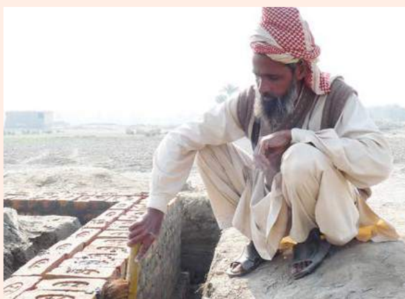
Mason pointing fired brick foundations for house reconstruction on raised platform in an effort to mitigate flood damage to the new house. The area has been affected by severe floods three times in ten years. Source: UN-Habitat.
