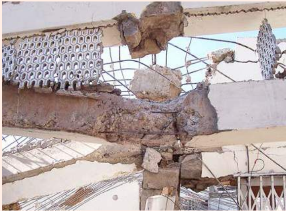
Damaged reinforced concrete building, impossible to repair and complex to retrieve salvage materials. Source: GOAL.
