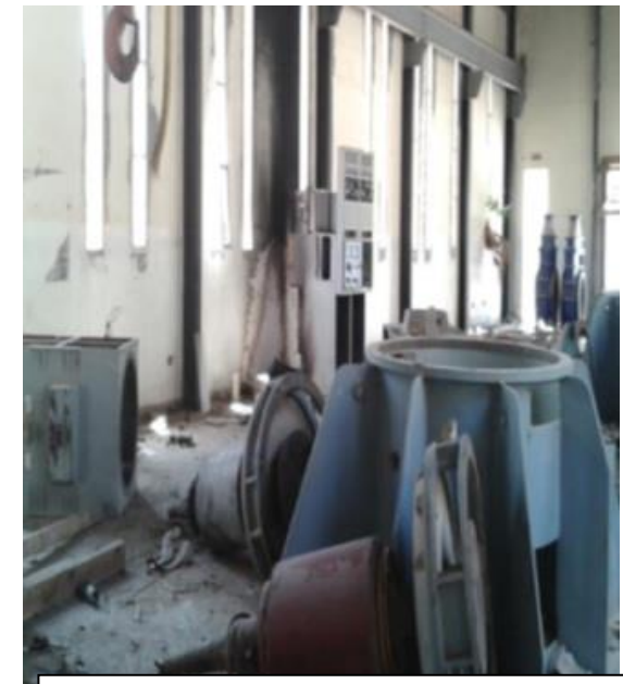
Damage in the main pumping station. Source: Key informants
