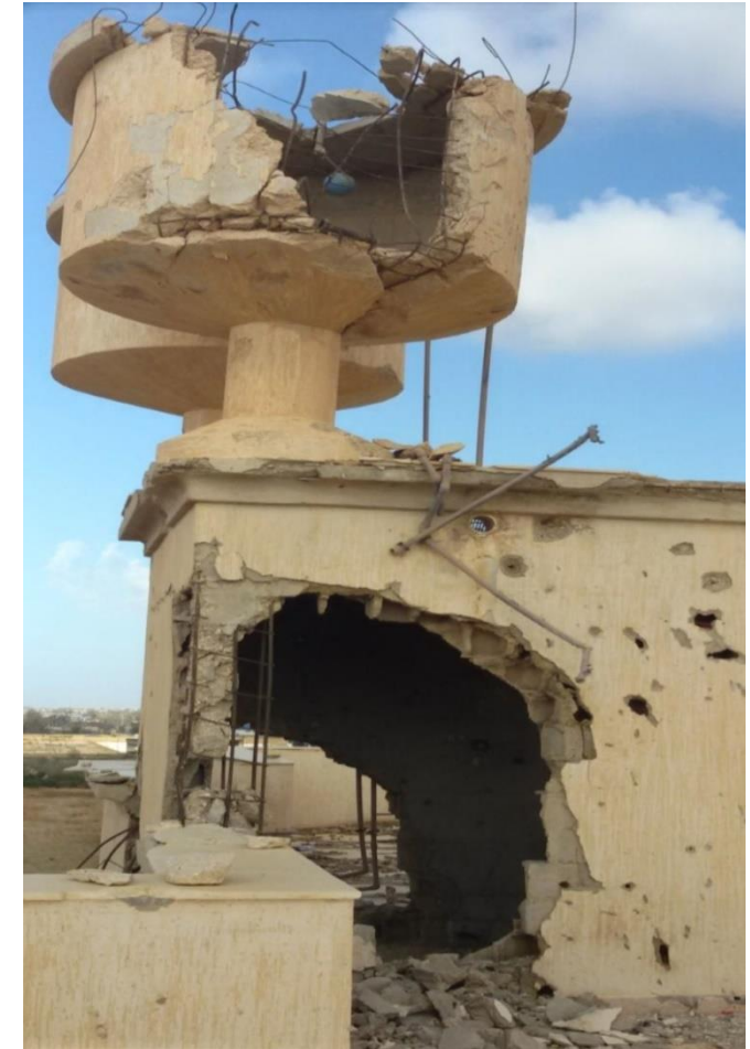
Damage in Benina services building, Courtesy: General Co for Water and Sanitation
