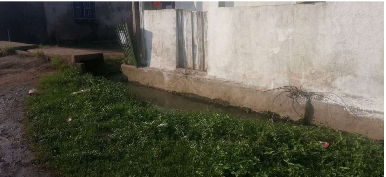
Photo 12. Stagnant water in a drainage channel. Source: UN-Habitat
