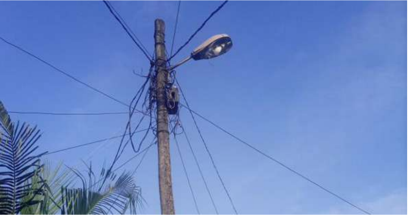
Photo 24. Street lights and power poles in Mambanda Source: UN-Habitat
