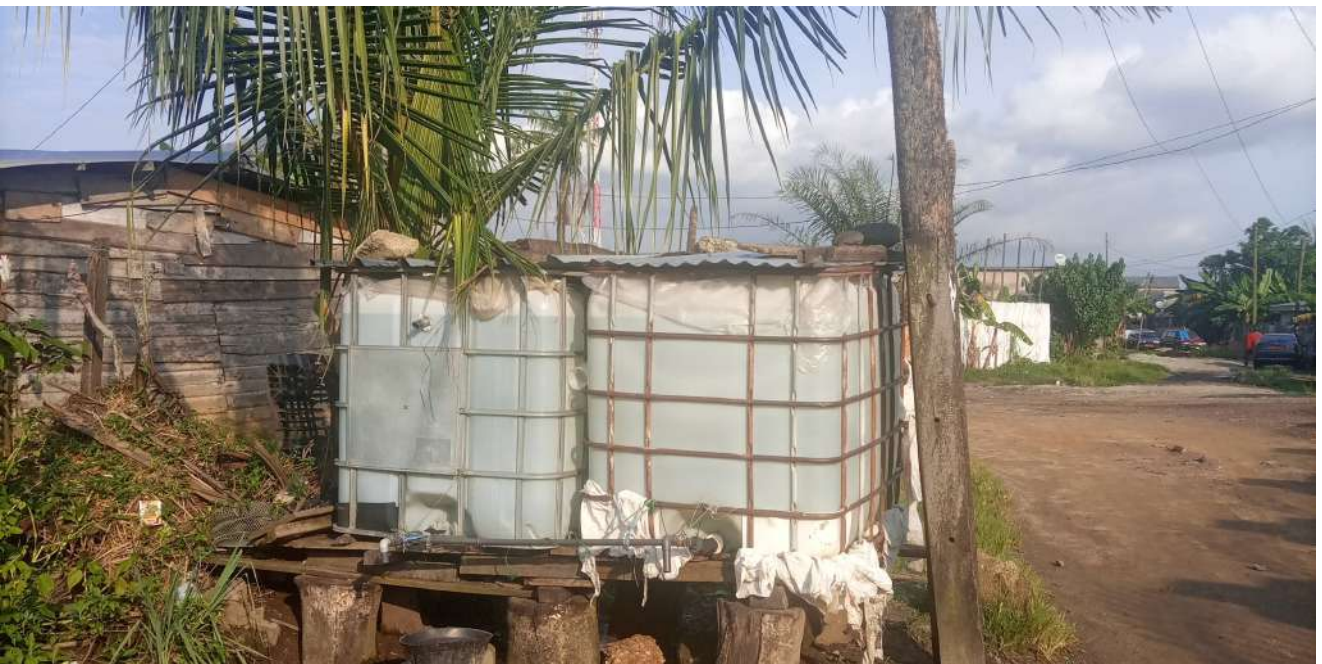
Photo 25. Private water fountains from which water is often sold Source: UN-Habitat
