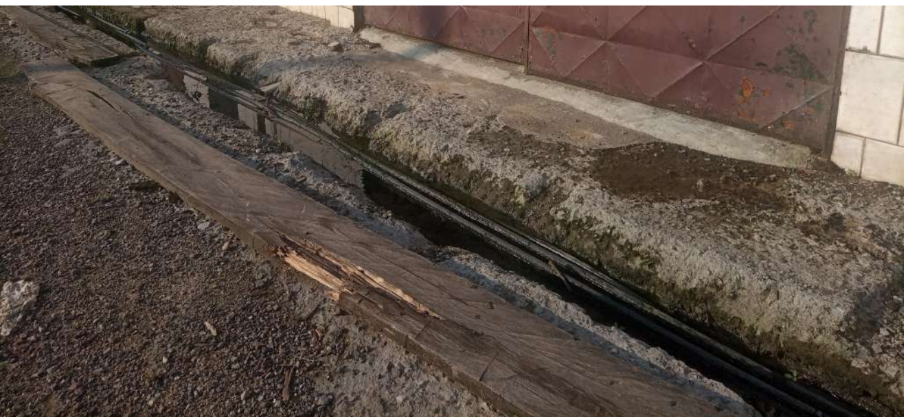
Photo 13. A rainwater drainage gutter. Source: UN-Habitat
