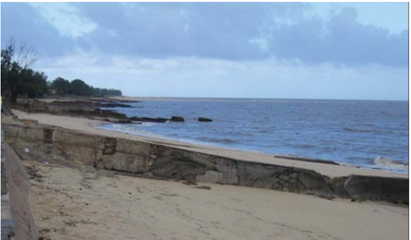
Beira; A deteriorated groyne 269
