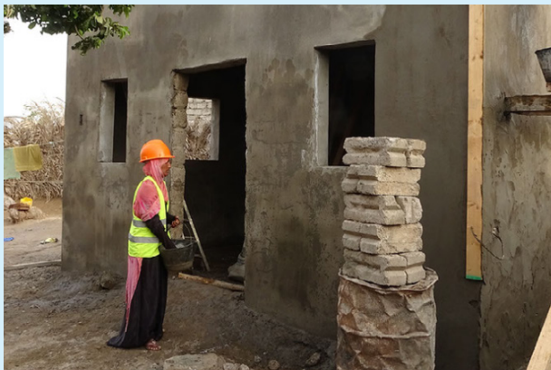
Figure 9: Housing and basic services rehabilitation in AlHudaydah-Yemen (before). Photo: © UN-Habitat
