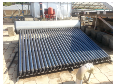
Solar water heater
