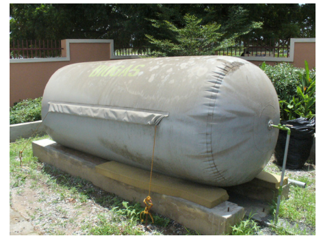
Above ground plastic inflatable gasholder
