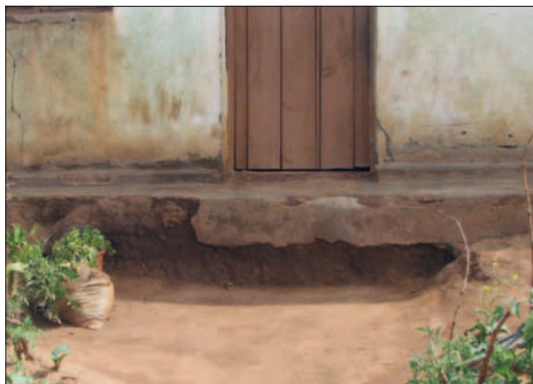
Figure 46. Insufficient foundations reduce the life of the building
