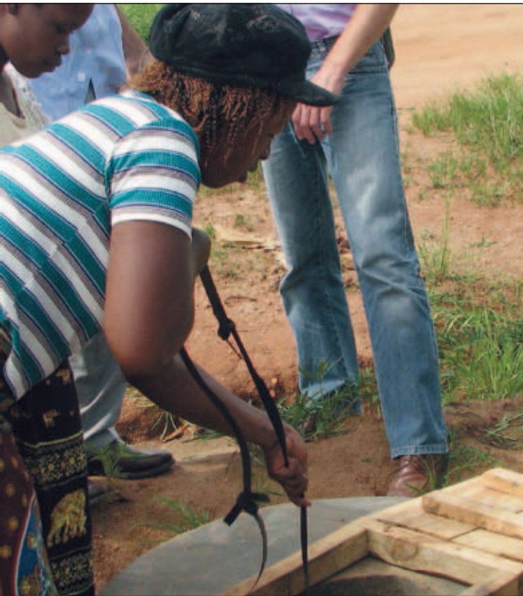
Figure 39. A shallow well in the CCODE estate, Area 49, Lilongwe Photo © Graham Tipple
