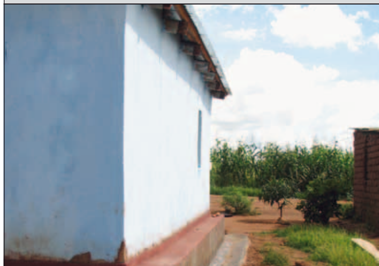
Figure 47. Good quality adobe walling, well plastered, high quality foundations and drainage and adequate roof overhand. CCODE Area 49, Lilongwe
