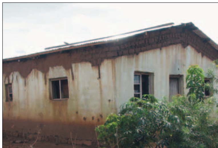
Figure 16. Roof failures in CCODE housing Area 49, Lilongwe have led to emergency repair and rebedding of roof tiles
