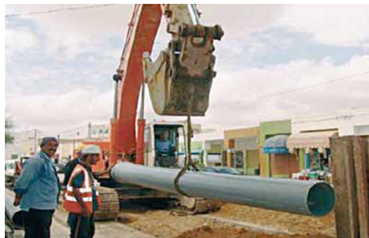
Figure 8.4 Installation of collector sewers Source: ONAS "akhbar el tathir" No. 14, page 8. December 2010.
