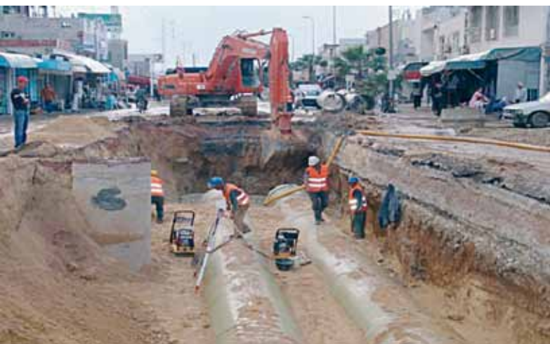
Figure 8.3 New sewerage main under construction Source: ONAS "akhbar el tathir" No. 14, page 5. December 2010.
