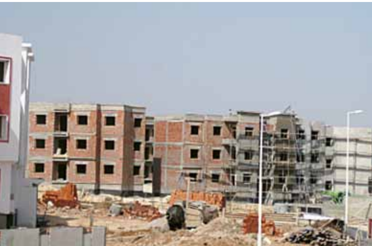
Figure 9.1 Example of construction in SNIT housing project, Sidi Hussain, Tunis Photo © Tarek El-Sheikh
