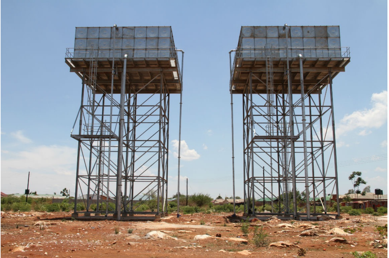
Figure 4.16: Tanks built to improve water reticulation in Woodlands Extension, Lusaka
