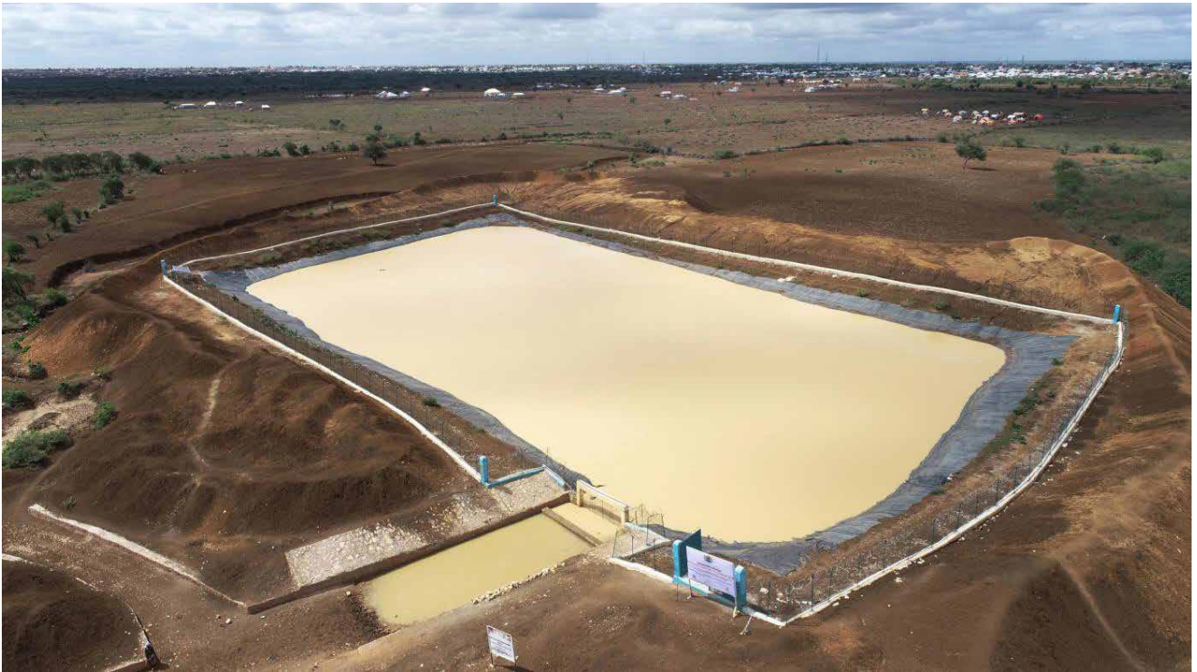
Fig. 31. Earthfill dam in Bonkai (Salamay Village) with a capacity of 25M litres ©NRC/Abdulkadir Mohamed
