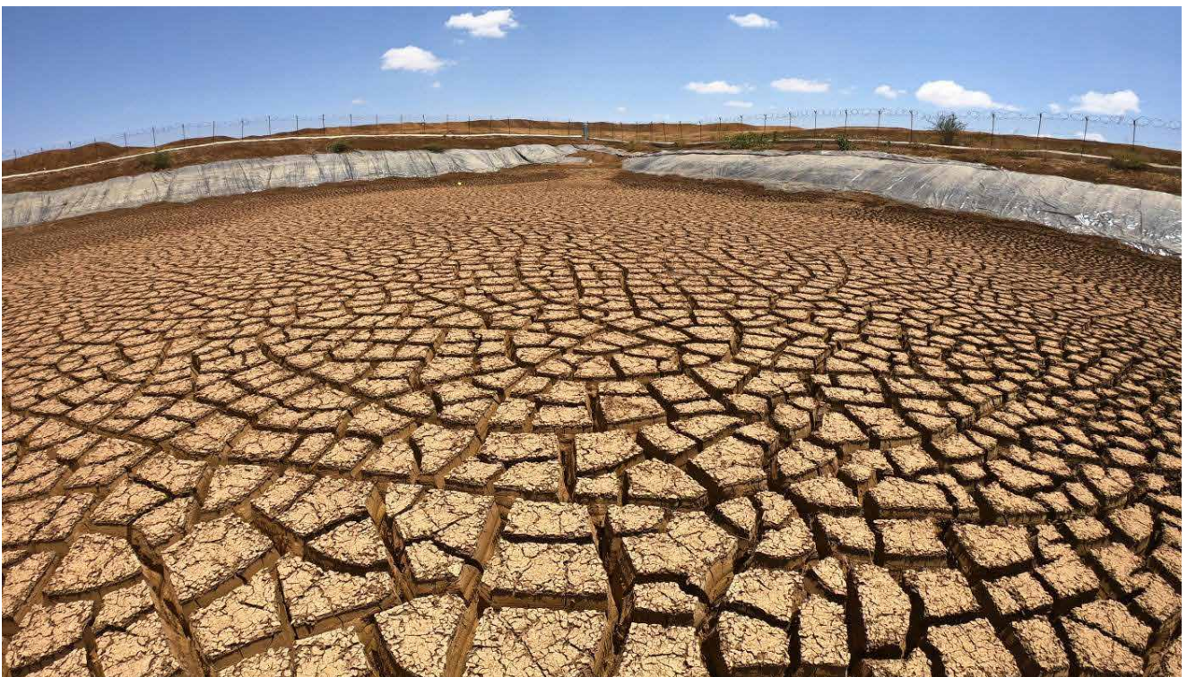
Fig. 32. The same dam in 2022, after three failed rainy seasons (Salamay Village) ©NRC/Will Seal
