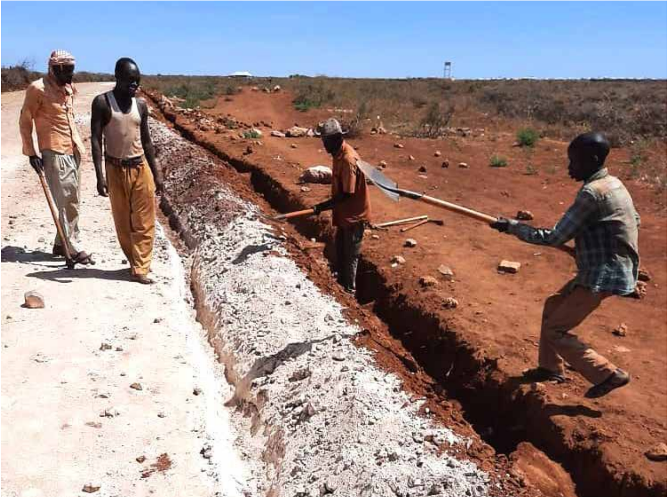
Fig. 55. Workers digging before installing drainage pipes along a newly constructed road © IOM
